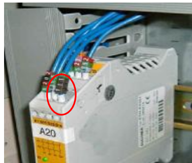
An example of a CCF where a single wire had been deliberately re-terminated to bypass a redundant pair of safety contacts resulting in a serious accident.
